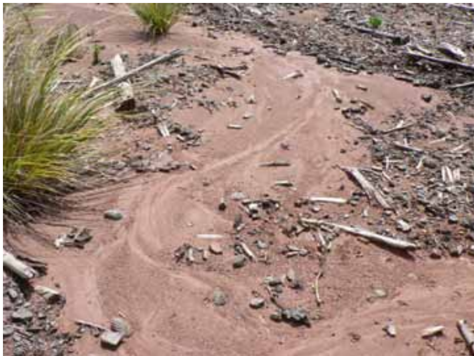
Site EP2: Close up view of the silt runoff from this skidder pad. The soil has a characteristic red colour and is coarse grained indicating loss of fine material when the area was clearfelled during harvest.
