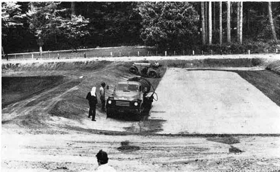
Grass carp ponds under construction on the Forest Research Institute campus. Because of the porous nature of the pumice soil the ponds were excavated and then sealed with bitumen.
