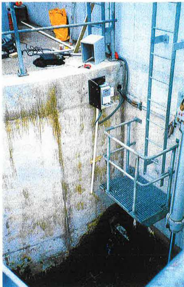
A Hydrologger / Microwire combination transmits a radial gate level reading as a 4–20 mA signal.
