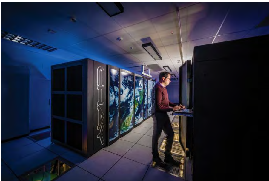
Three Cray supercomputers make up the High Performance Computing Facility. Together they are capable of processing more than two thousand trillion calculations per second. [Dave Allen]
