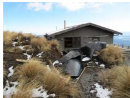
Damage to Ketetahi Hut following the Tongariro eruption. Photo: Brad Scott, GNS Science.
