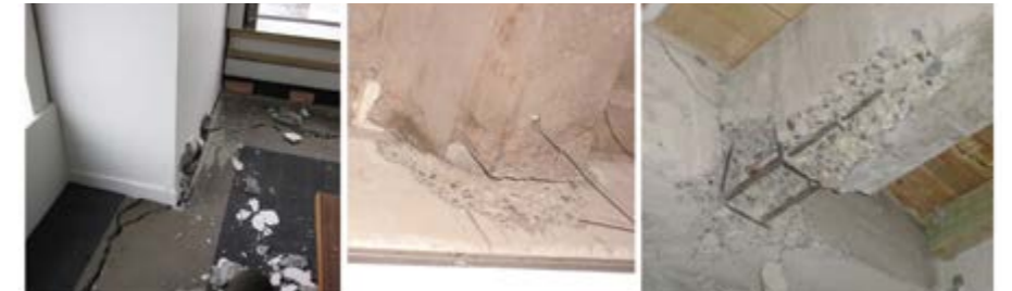
Figure 1: Damage to precast floors during the Canterbury earthquakes
