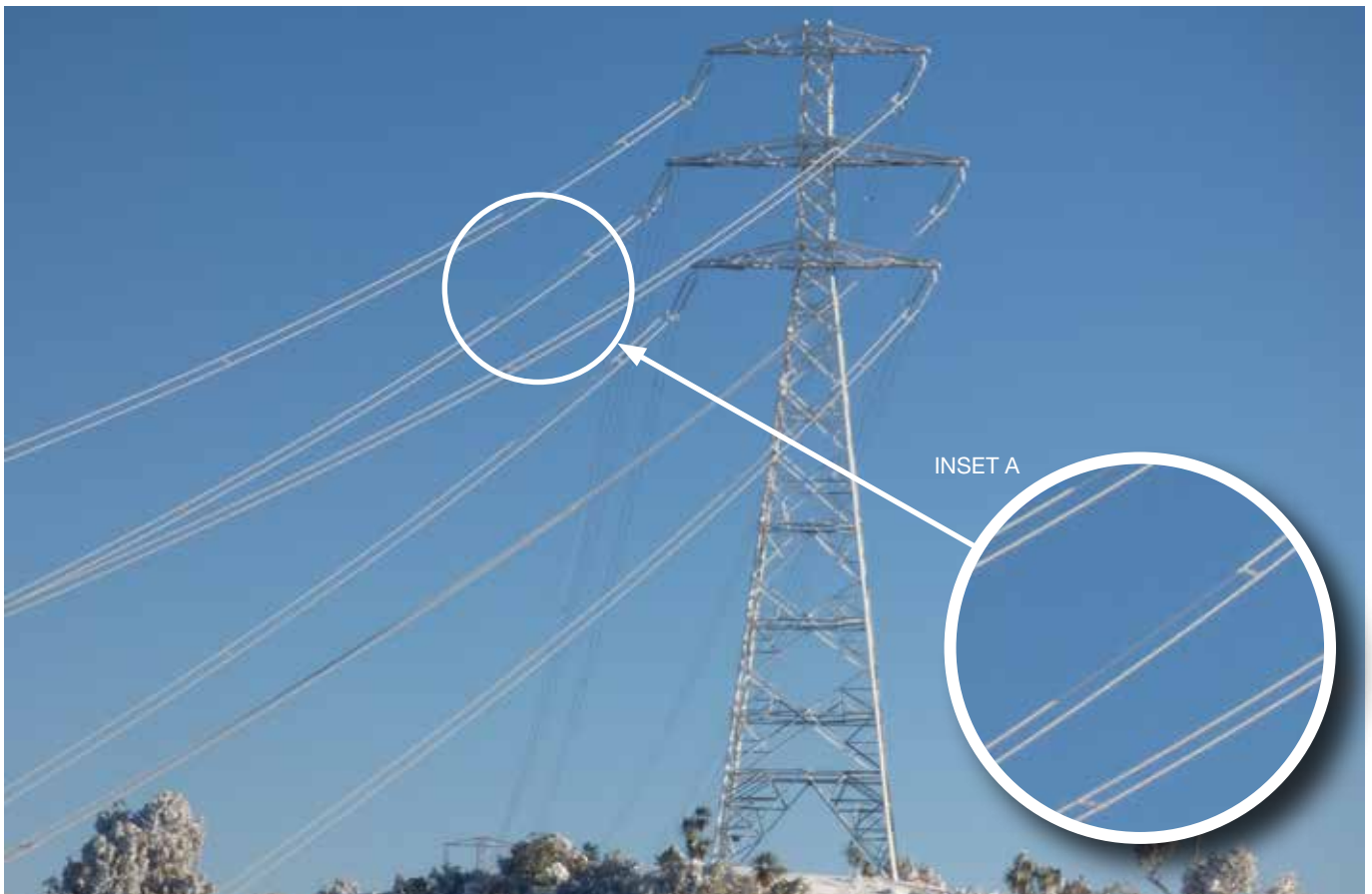
Fig. 2. Snow and Ice accretion (INSET A) on a high elevation span of HVDC line WRK-WHI-A on 7 August at the eastern edge of Rangitaiki plain. Photo: Alan Lyne, Transpower.
