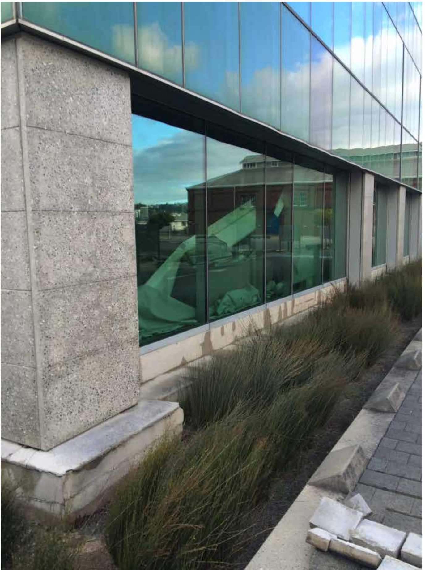
Damage to Statistics House following the 2016 Kaikōura earthquake. Photo: Statistics New Zealand.
