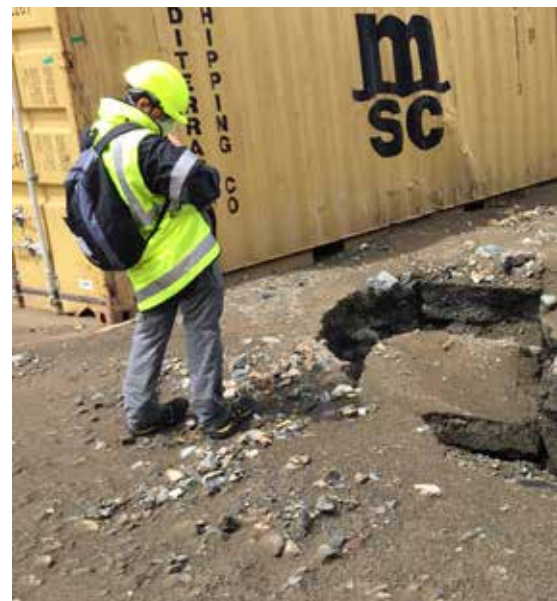
Liquefaction at CentrePort following the 2016 Kaikōura earthquake. Photos: University of Canterbury.
