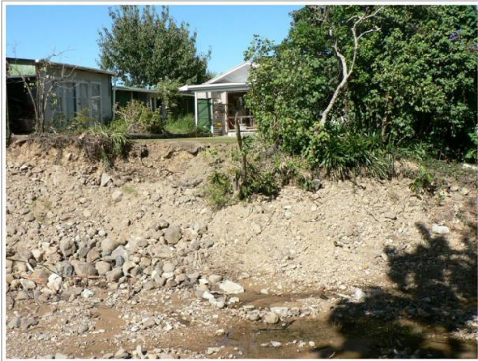
2 Erosion outside 624 Thames Coast Rd
