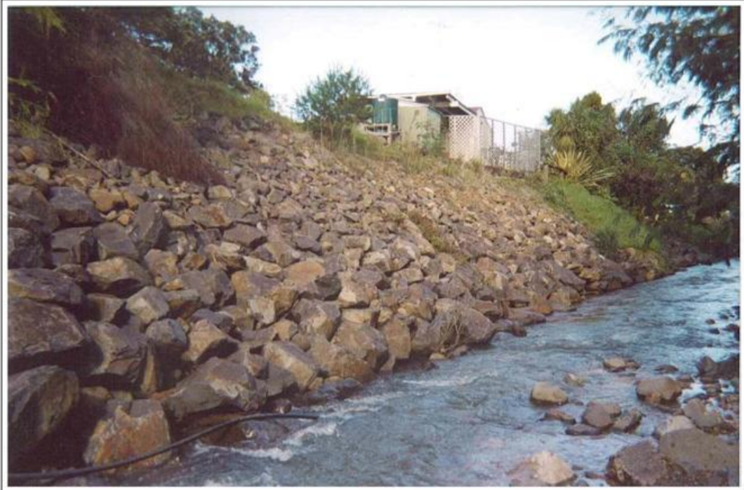
1 Erosion protection outside 7 Valder Place
