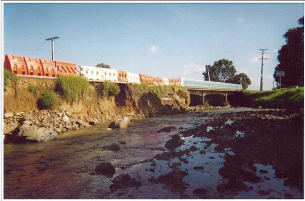
3. Erosion of left bank at SH 25 bridge
