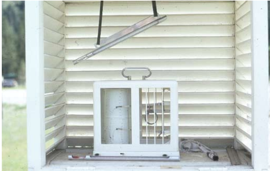
Figure 9. Hygrothermograph mounted in separate screen with double-louvered sides and double roof. Photo courtesy of British Columbia Ministry of Forests and Range, Protection Branch.
