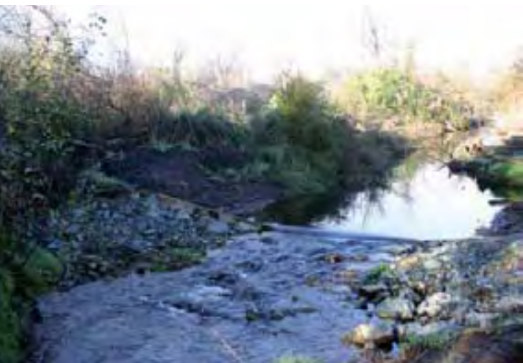
Water control structure on the outlet of Lake Rotomanuka North. Photo courtesy of Environment Waikato.
