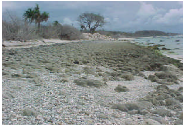
Figure 3. Beach morphology and erosion. Note exposed dolomite substrate on the lower beach and erosion at beach-land interface.
