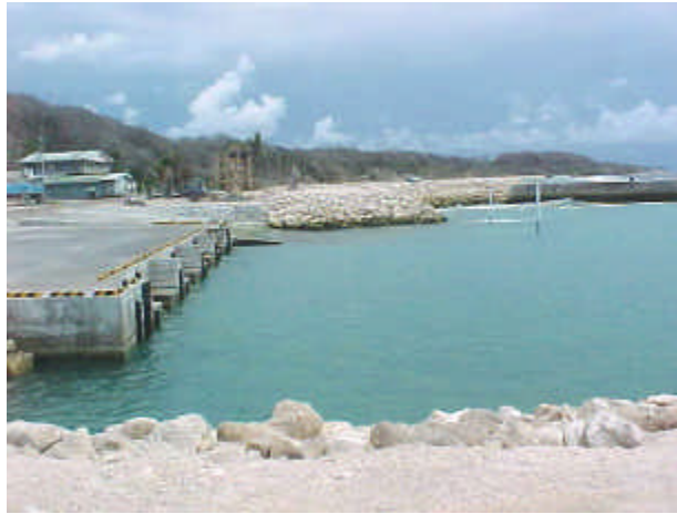
Figure 2. The harbour. Left – mooring basin/wharf, with quay wall and apron; top right – sub-breakwater; top center – rubble groin with rip-rap spending slope, lower center – rubble groin.
